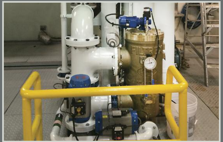
ACB filters in operation
