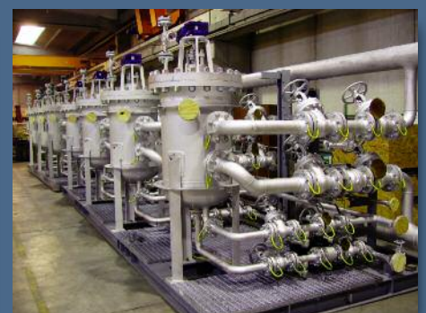
Feed Filter for Hydrocracker Unit (VGO) – Bangkok, Thailand
