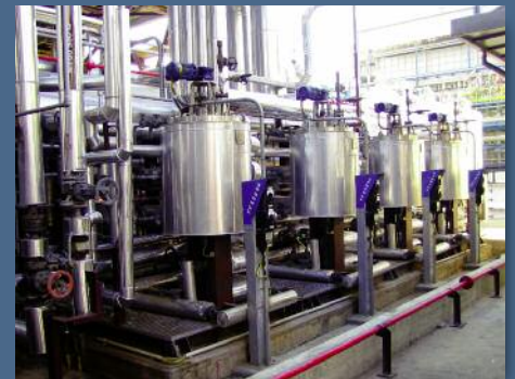
Feed Filter for CR-40 DAO GOFINER Unit (Deasphalted Oil) Priolo Gargallo, Italy
