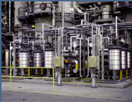
Feed Filter for Hydrocracker Unit (Blend of HCGO/HVGO) Port Arthur, USA
